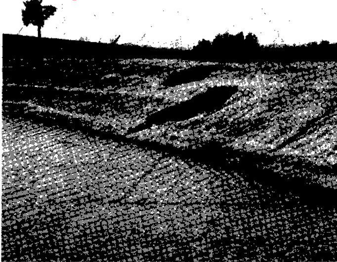
Figure 8.1. Examples of piping failure of a dam due to the presence of dispersive soils (Soil Conservation Service of NSW).
